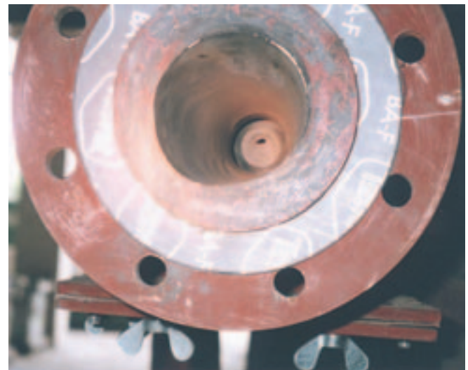
Fig. 2: Erosion by high-wear coarse ash on a steel diffusor after transport
